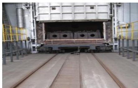
Large-scale Car Tape Gas Heating Furnace
