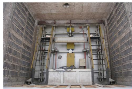
Take off the trolley furnace
